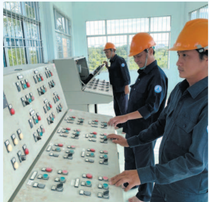
Technicians are operating the water plant
