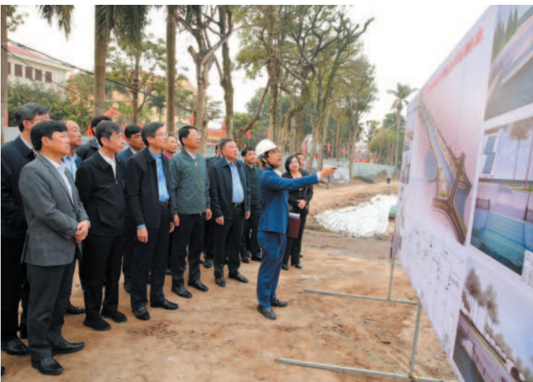
Ninh Binh Provincial Party Secretary Doan Minh Huan, accompanied by a working delegation, conducts a survey of the progress on the Nam Song Van Irrigation Cluster project, Feb 2024
